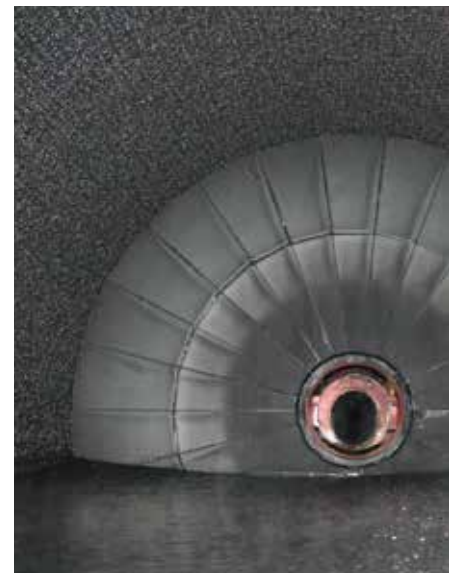
Metso develops tailor-made lining systems with focus on function, lifetime, and rapid installation.
