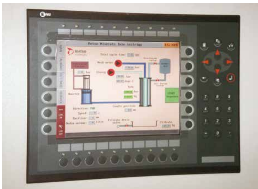
Typical operator interface
